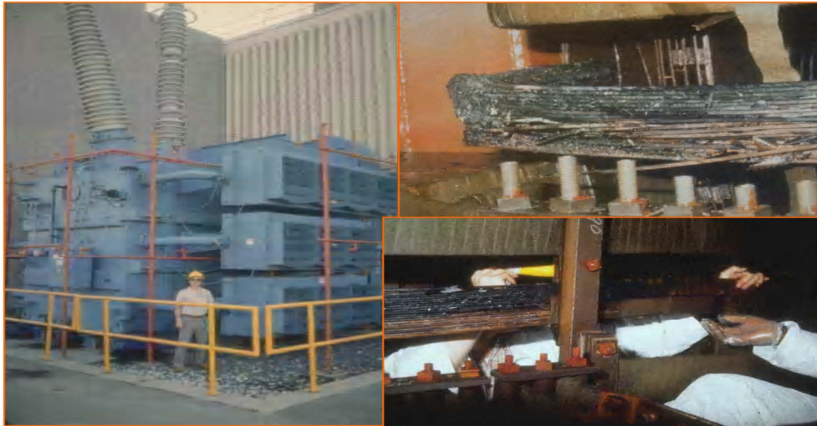
Figure 2-33. Damaged transformer at the Salem Nuclear Plant.
